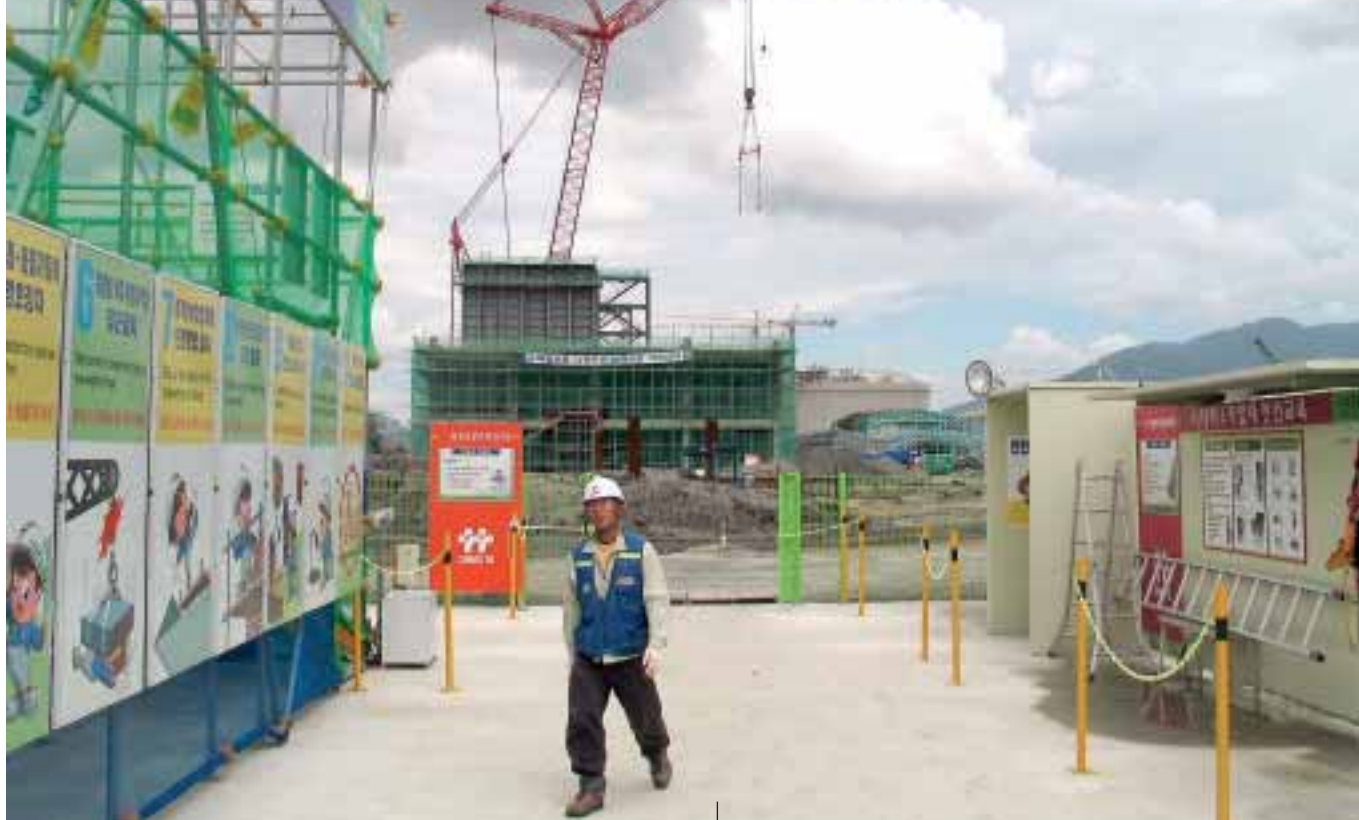
Daelim has developed a method for communicating what are safe and what are poor working practices on their construction site, which was considered as "best-in-class" in a recent audit by DNV.
